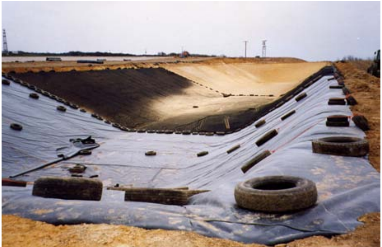
Photo3: Lining in sandy sub- strate
